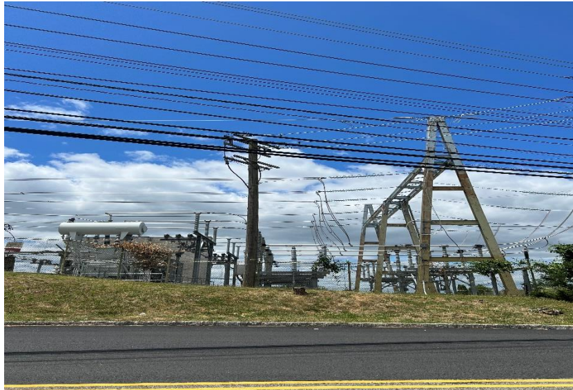
Figure 3: View of switching equipment from the north of the site
