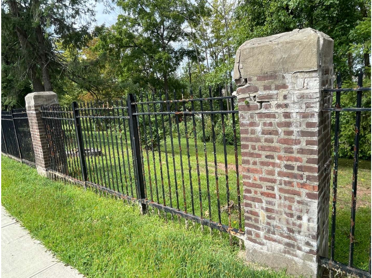
View of station fence along Prospect Avenue, taken August 28, 2024, showing rusting fence sections and deteriorating brick pillars.
