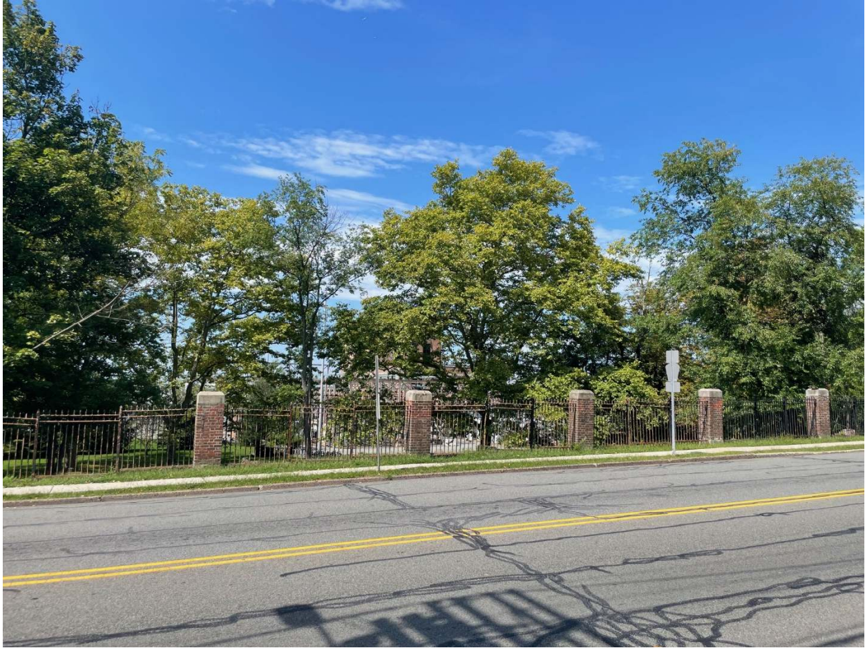
View of station fence along Prospect Avenue, taken August 28, 2024, showing rusting fence sections. A lightning mast is shown behind the trees.
