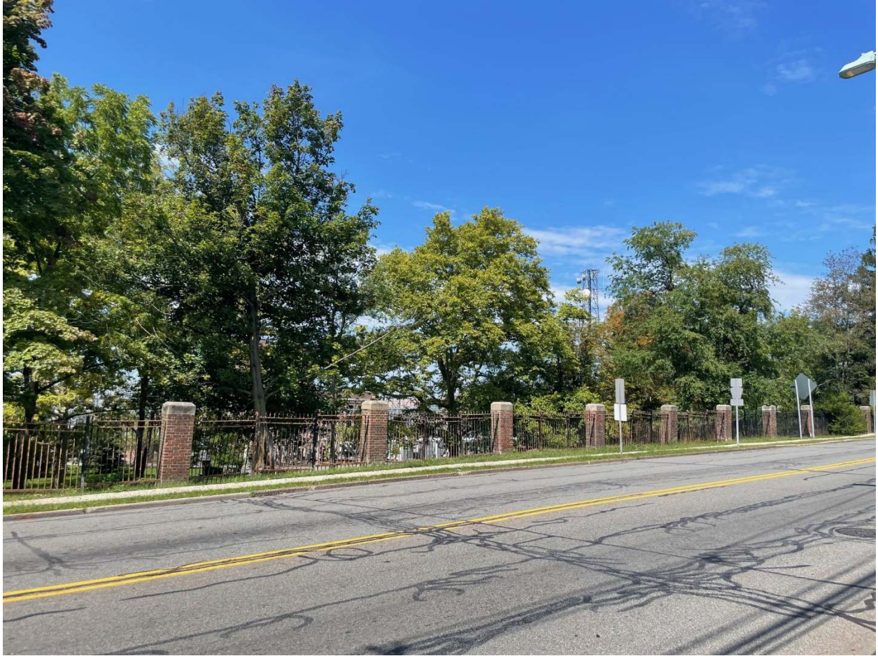
View of station fence along Prospect Avenue, taken August 28, 2024, showing rusting fence sections. PSE&G's microwave/radio tower is shown on the right side behind the trees.
