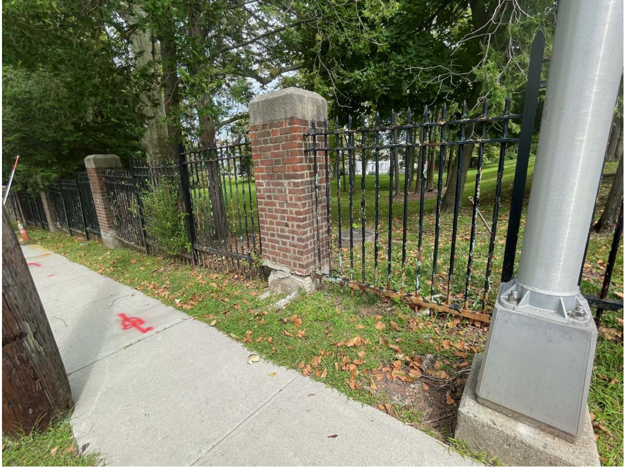
View of station fence on Mount Pleasant Avenue at the intersection of Mount Pleasant Avenue and Prospect Avenue, taken August 28, 2024, showing rusting fence sections and deteriorating brick pillars.
