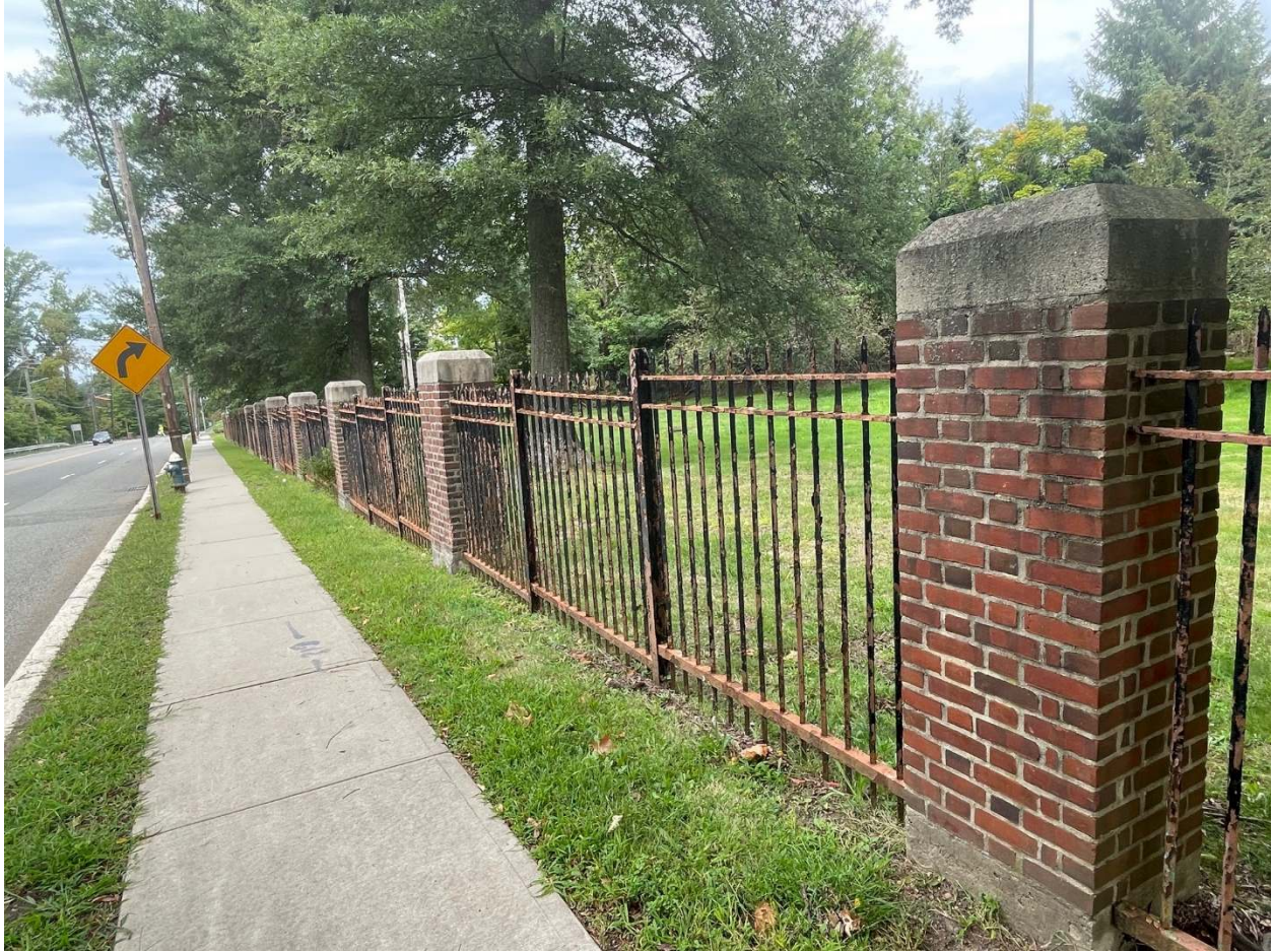
View of station fence along Prospect Avenue, taken August 28, 2024, showing rusting fence sections and deteriorating brick pillars, with a lightning mast in the background.
