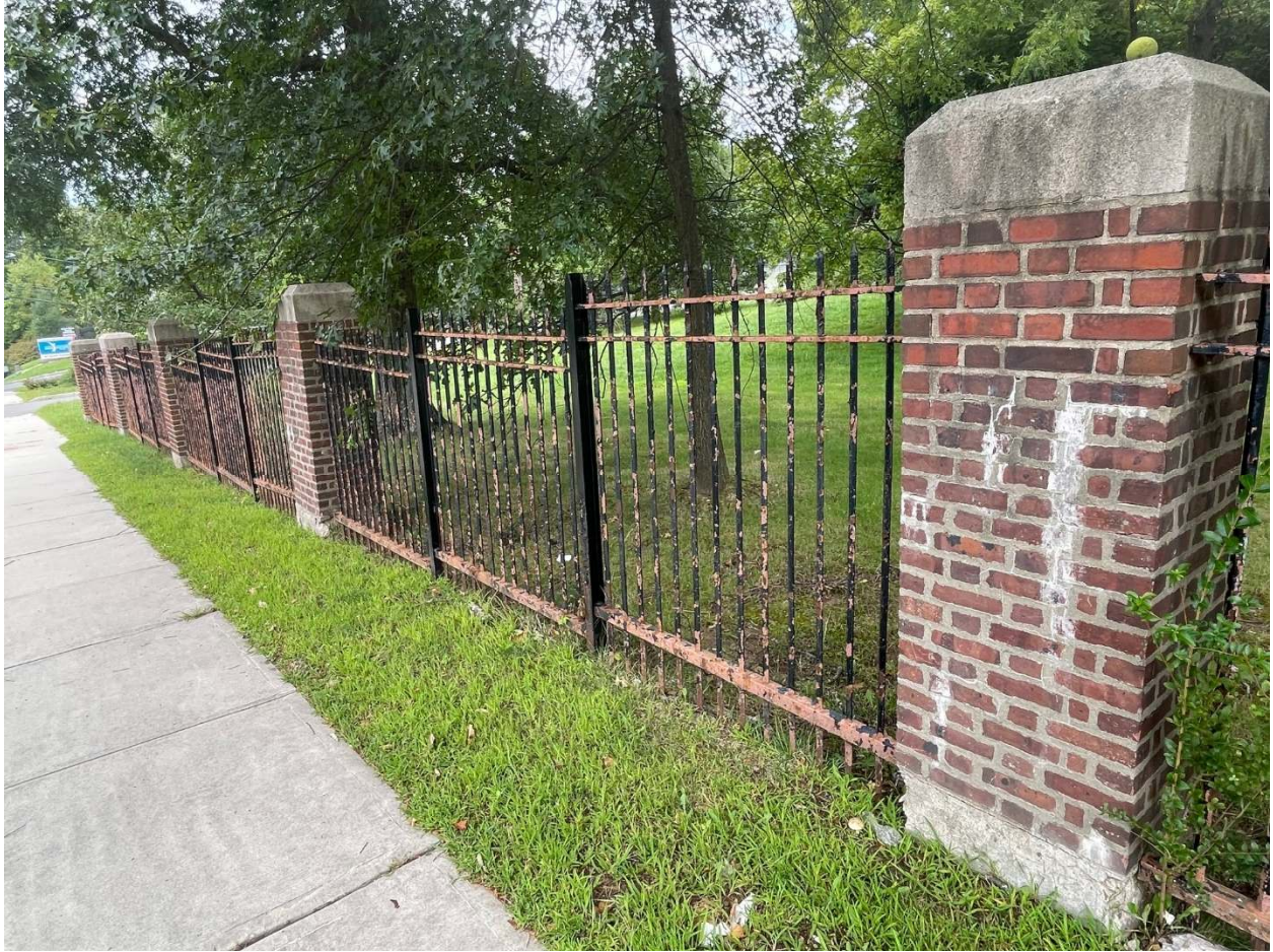
View of station fence along Mount Pleasant Avenue look west, taken August 28, 2024, showing rusting fence sections.
