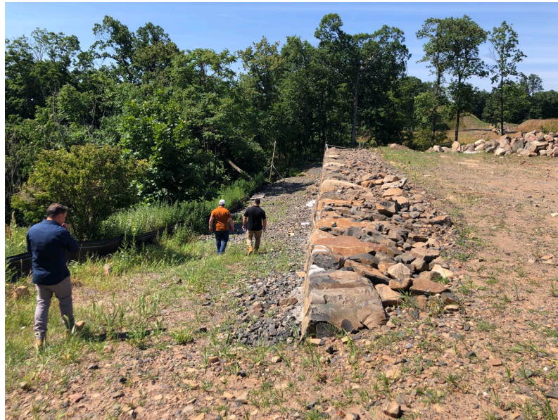
Again, due to heavy rainfall and thunderstorms, the 15' buffer between the east side of the wall and the downstream property line, should be restored to grade, along with addition of crushed stone, thereby removing the potential for erosion. This cannot be done unless the contractor simultaneously removes the top temporary portion of the retaining wall, which will then result in the wall complying with the allowable height. Colliers recommends a full-time inspector from our office be on site to ensure proper construction means and methods are followed, and an additional interim as-built be performed to confirm the finished wall doesn't exceed 6' in any area and that it conforms to the Matarazzo plans submitted to the Township.
