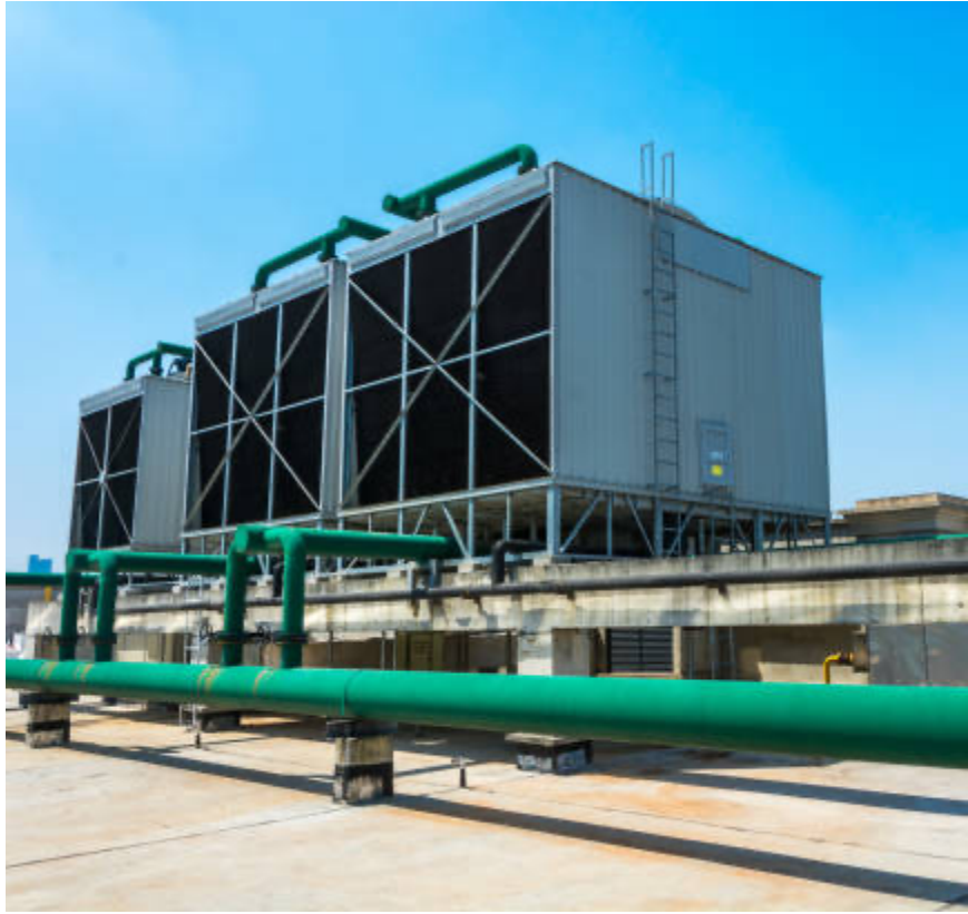
Cooling towers approximately 1500 tons
