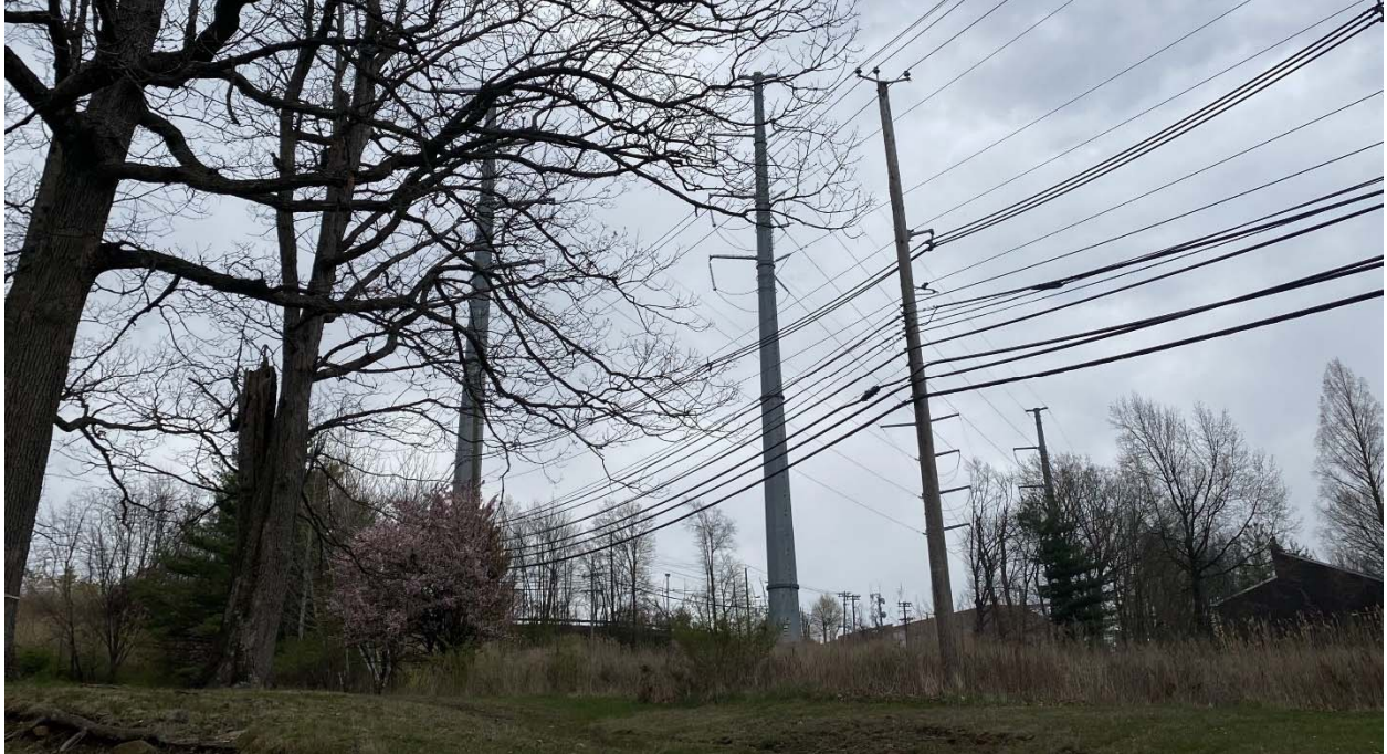
PSE&G electric transmission lines on Block 155, Lot 26.01
