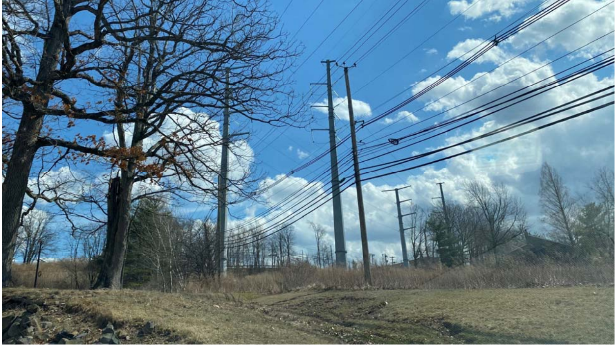
PSE&G electric transmission lines on Block 155, Lot 26.01
