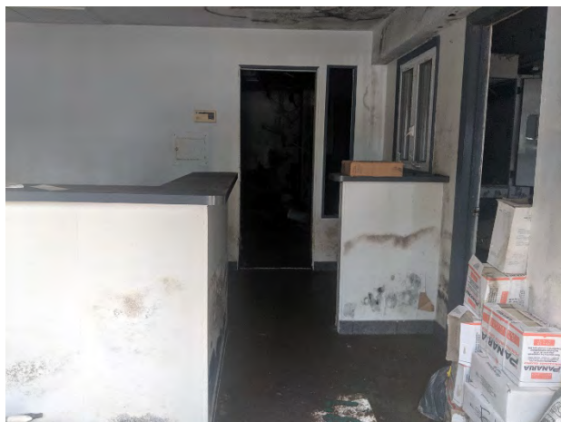
Auto Body Office - Water Damage
