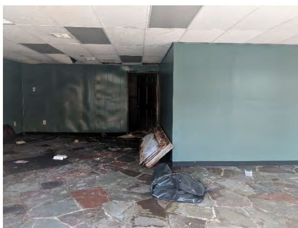
Corner Retail Space - Debris and Damage - Water Damage & Ceiling Tiles Warping
