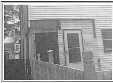
Missing Siding / Deferred Maintenance
