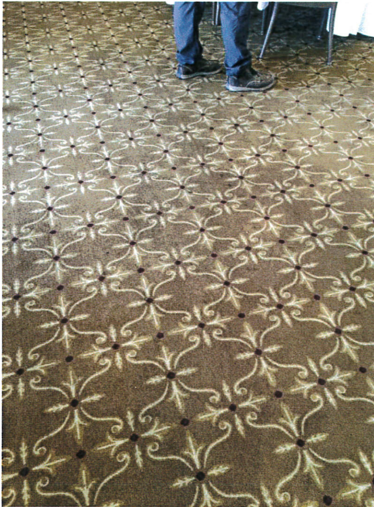
106 106-Pre-Mitigation - Dining Room Date Taken: 12/26/2022 (Zone 1) 3
