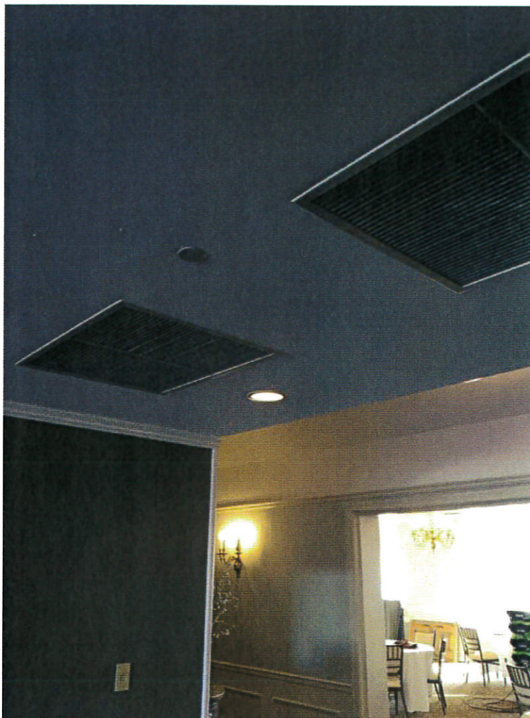
120 120-Pre-Mitigation - Foyer (Zone 2) Date Taken: 12/26/2022 3
