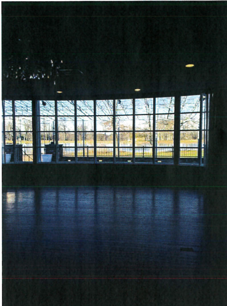
97 97-Pre-Mitigation - Ball room Date Taken: 12/26/2022 (Zone 2) 7
