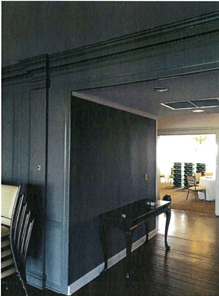
92 92-Pre-Mitigation - Ball room Date Taken: 12/26/2022 (Zone 2) 2
