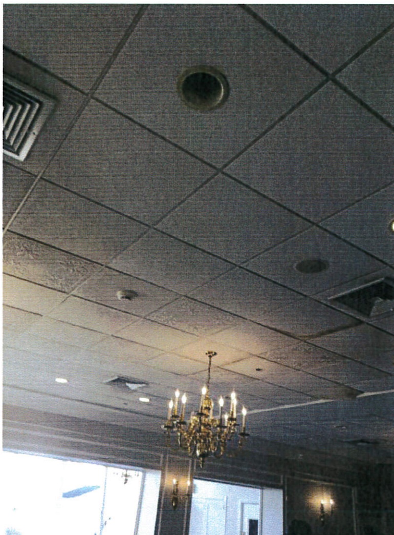
102 102-Pre-Mitigation - Dining Room Date Taken: 12/26/2022 (Zone 1) 11
