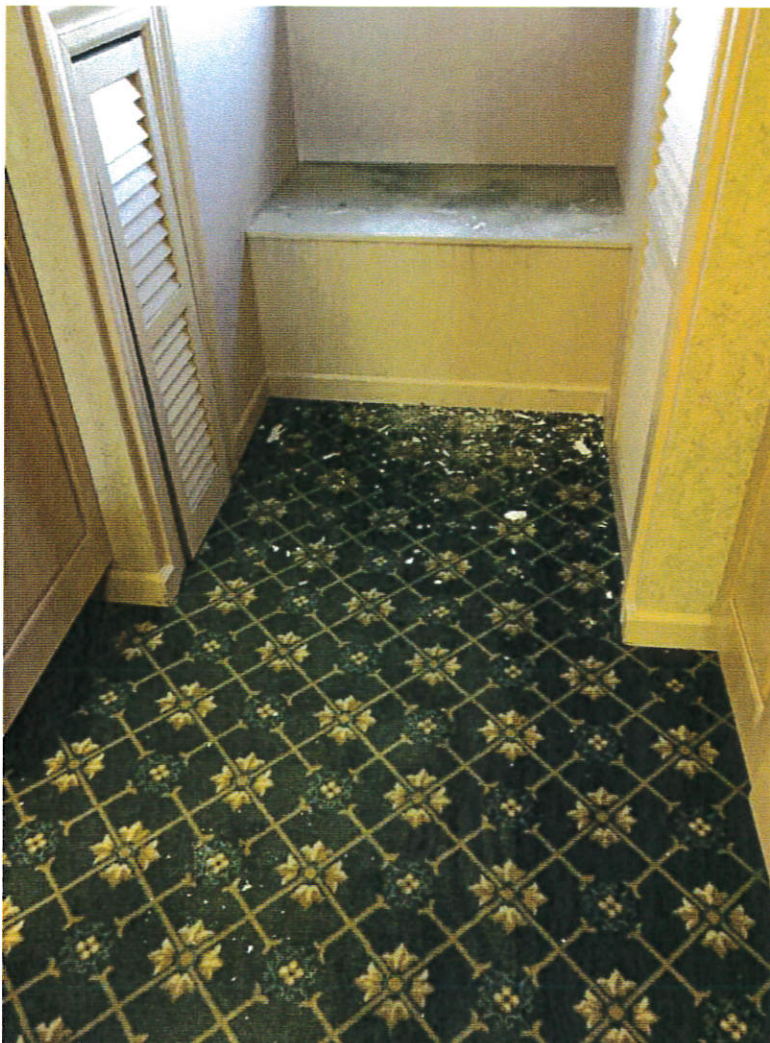
144 144-Pre-Mitigation - Locker room Date Taken: 12/26/2022 (Zone 1) 14
