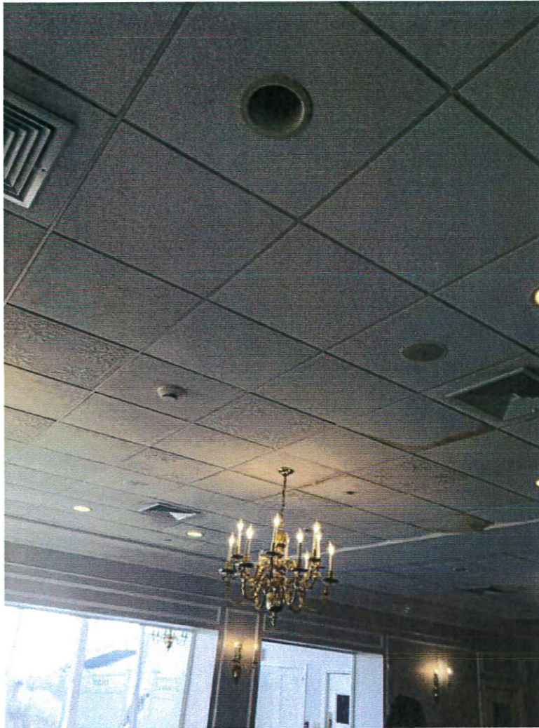
101 101-Pre-Mitigation - Dining Room Date Taken: 12/26/2022 (Zone 1) 10
