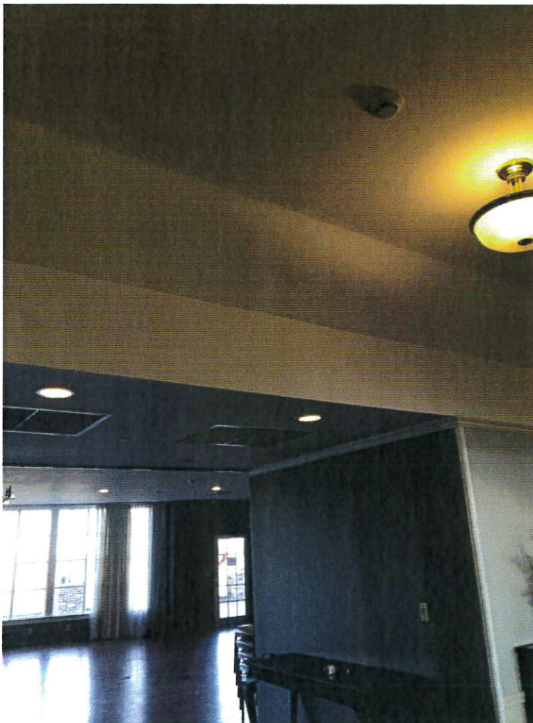
114 114-Pre-Mitigation - Foyer (Zone 2) Date Taken: 12/26/2022 10
