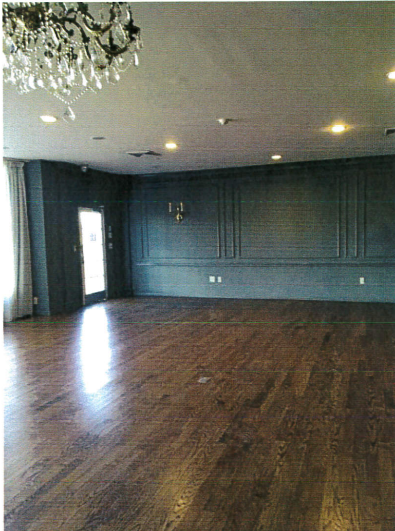
99 99-Pre-Mitigation - Ball room Date Taken: 12/26/2022 (Zone 2) 9
