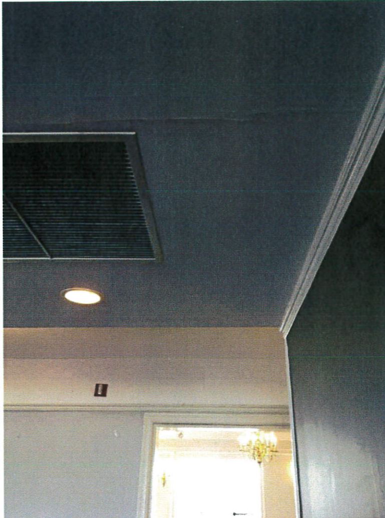
121 121-Pre-Mitigation - Foyer (Zone 2) Date Taken: 12/26/2022 4
