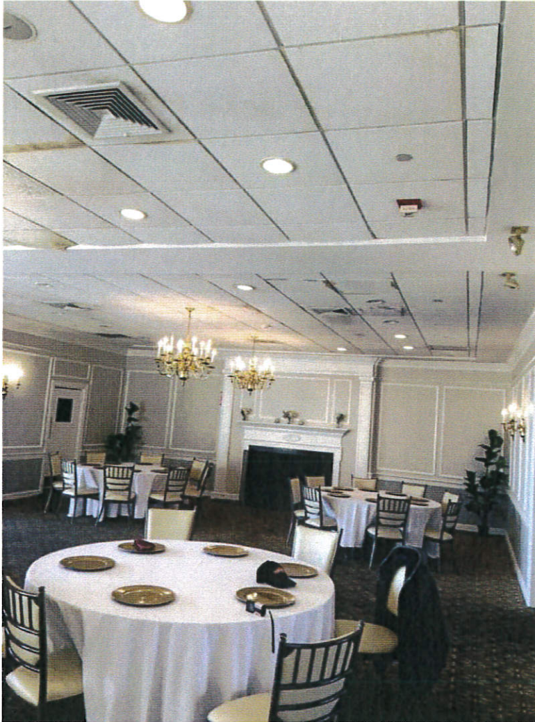
112 112-Pre-Mitigation - Dining Room Date Taken: 12/26/2022 (Zone 1) 9
