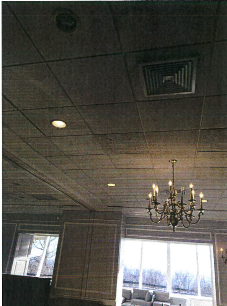
103 103-Pre-Mitigation - Dining Room Date Taken: 12/26/2022 (Zone 1) 12
