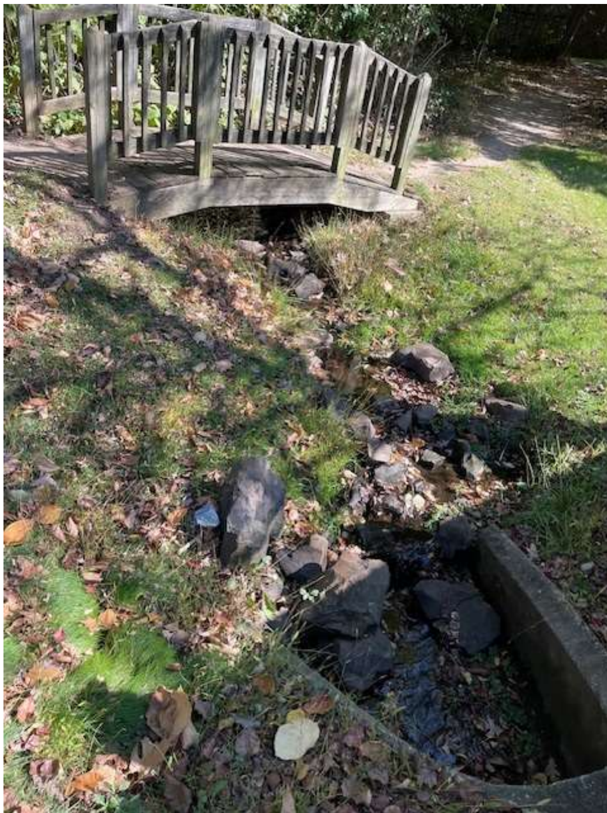
OUTFALL FLARE END SECTION FOR LAKE BY PEDESTRIAN BRIDGE
