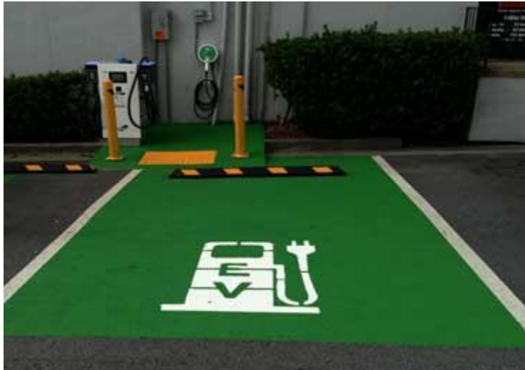
Electric Vehicle Charging Station
