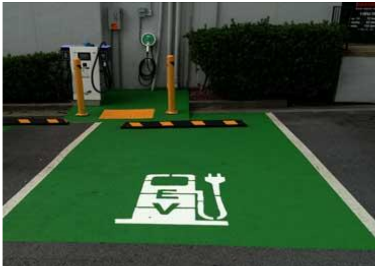
Electric Vehicle Charging Station
