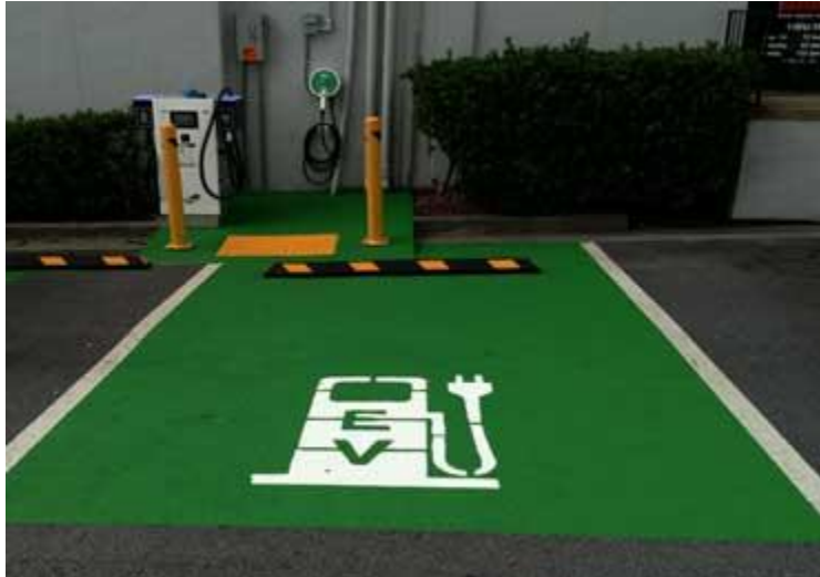
Electric Vehicle Charging Station
