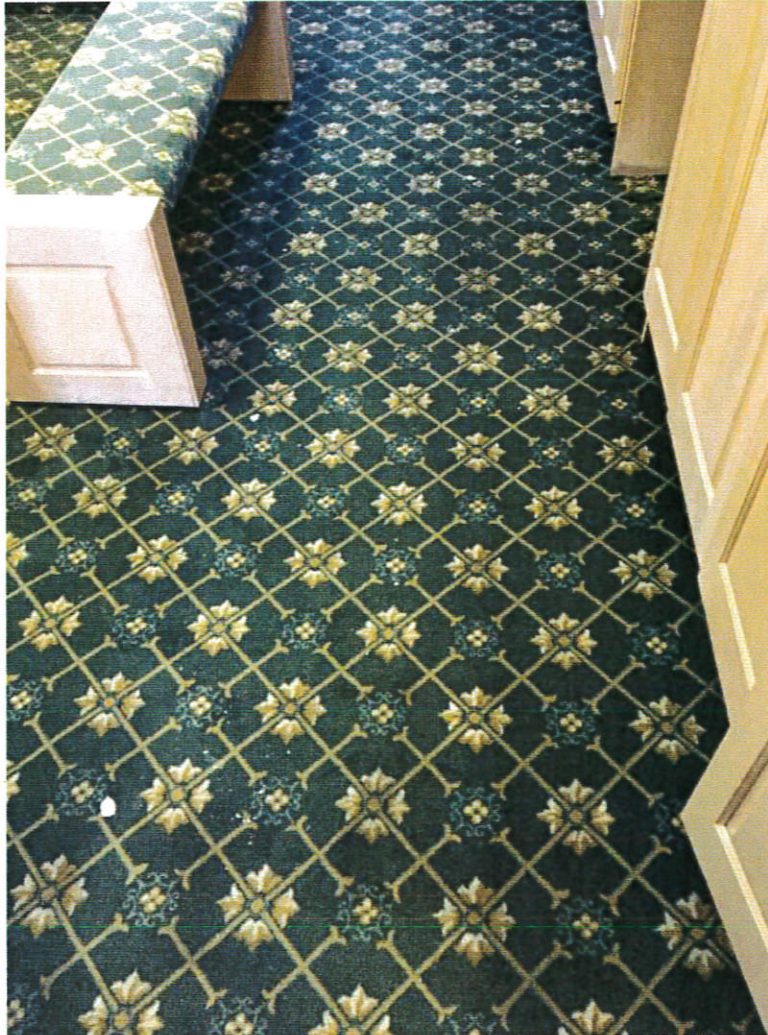
145 145-Pre-Mitigation - Locker room Date Taken: 12/26/2022 (Zone 1) 15
