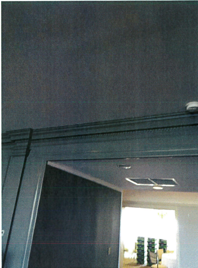
93 93-Pre-Mitigation - Ball room Date Taken: 12/26/2022 (Zone 2) 3
