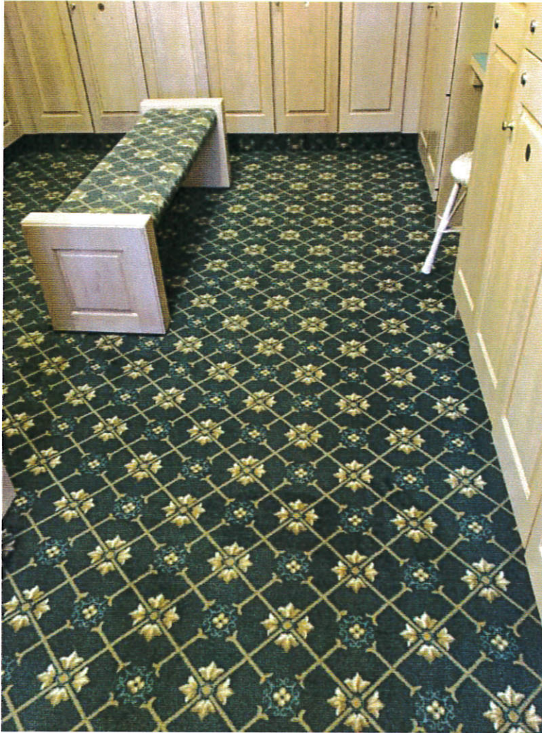
150 150-Pre-Mitigation - Locker room Date Taken: 12/26/2022 (Zone 1) 4
