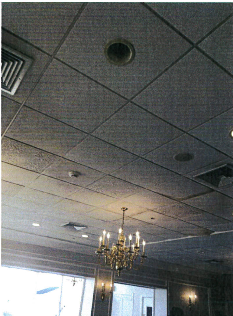
102 102-Pre-Mitigation - Dining Room Date Taken: 12/26/2022 (Zone 1) 11
