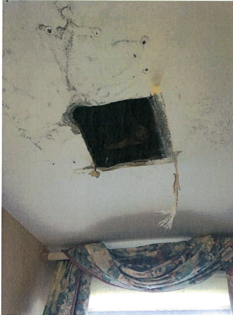
142 142-Pre-Mitigation - Locker room Date Taken: 12/26/2022 (Zone 1) 12
