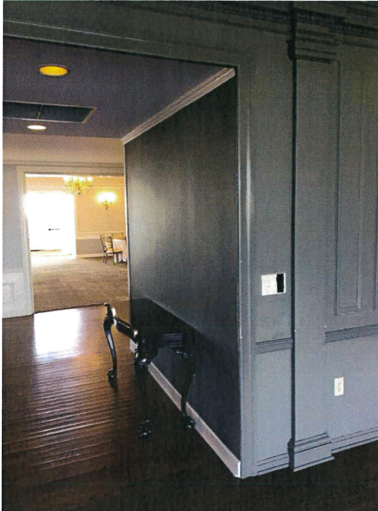
122 122-Pre-Mitigation - Foyer (Zone 2) Date Taken: 12/26/2022 5
