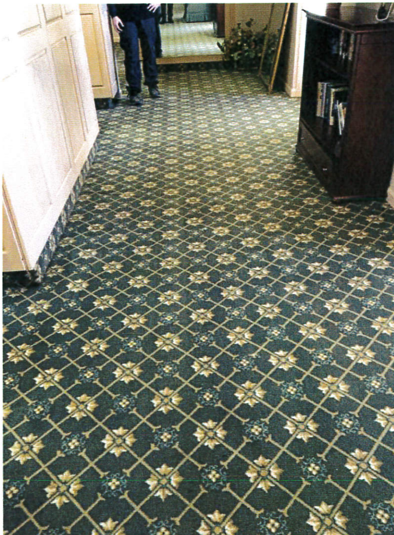
153 153-Pre-Mitigation - Locker room Date Taken: 12/26/2022 (Zone 1) 7
