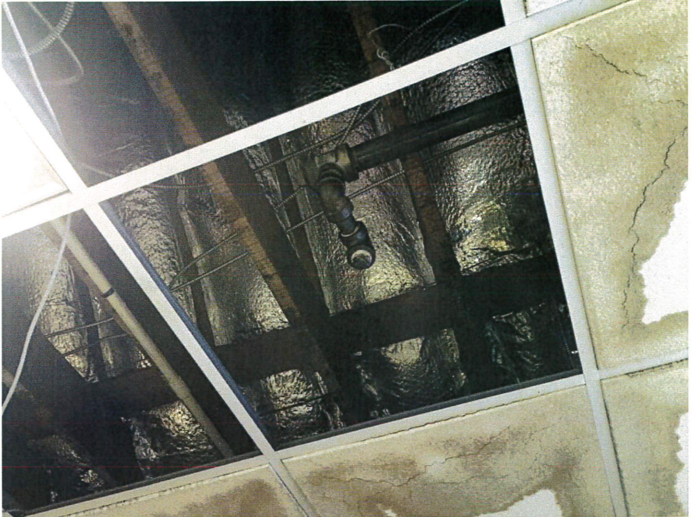
1 1-Cause of LossSource of Damage Date Taken: 12/26/2022
