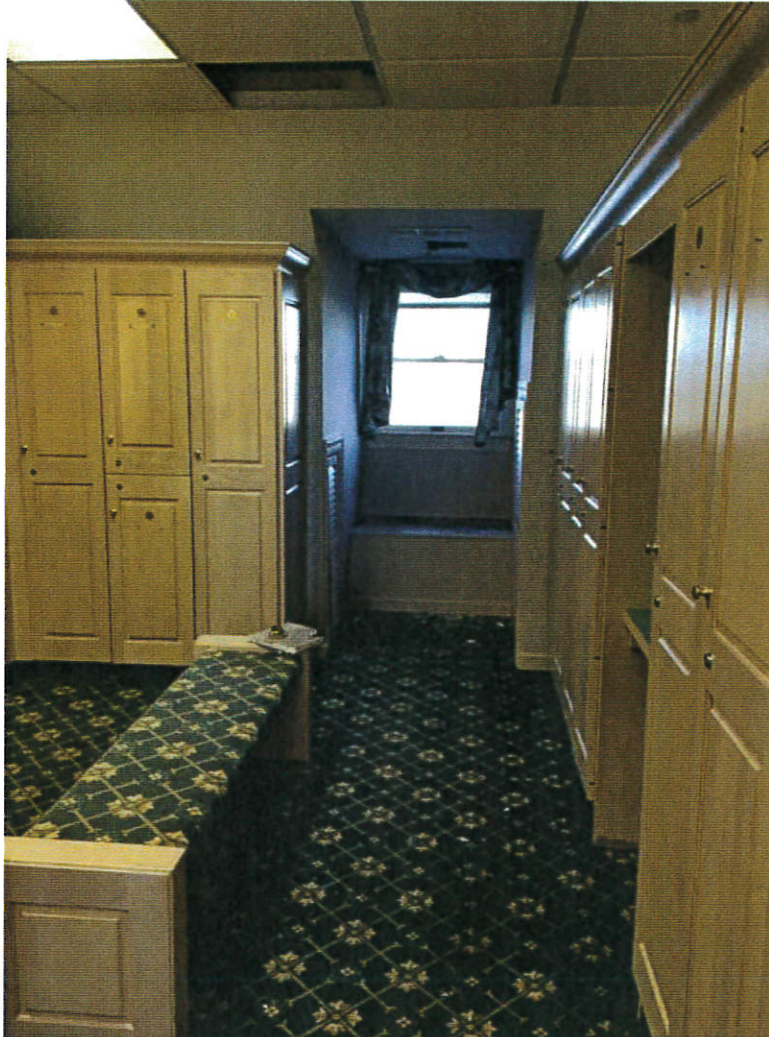
146 146-Pre-Mitigation - Locker room Date Taken: 12/26/2022 (Zone 1) 16
