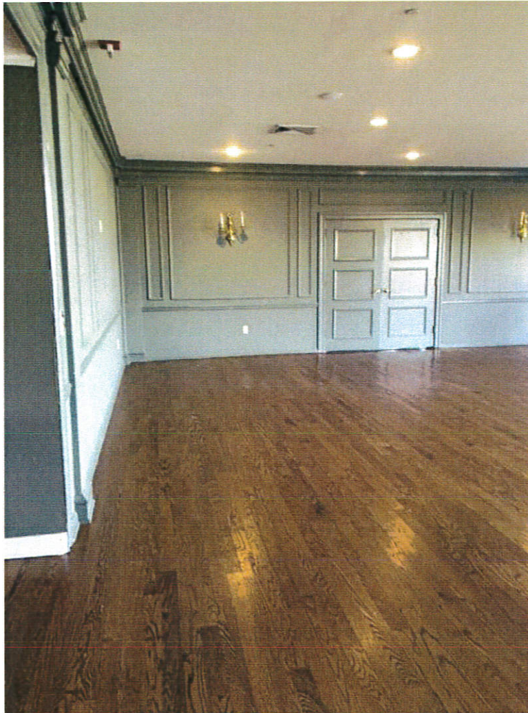
95 95-Pre-Mitigation - Ball room Date Taken: 12/26/2022 (Zone 2) 5
