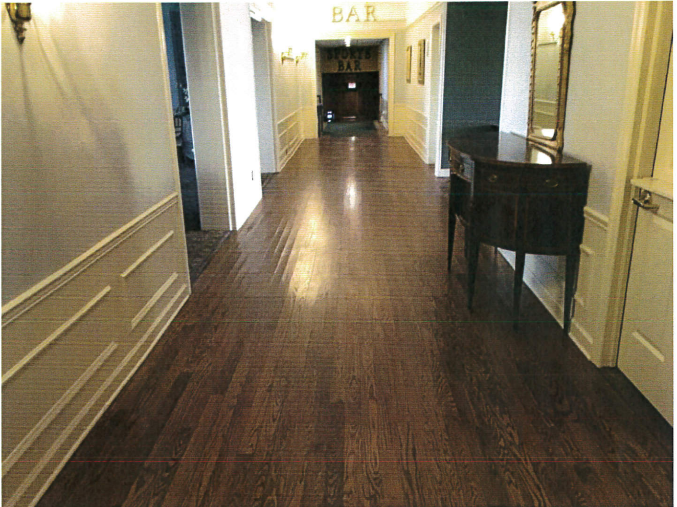
71 71-Post Mitigation - Foyer (Zone 2) Date Taken: 12/30/2022
