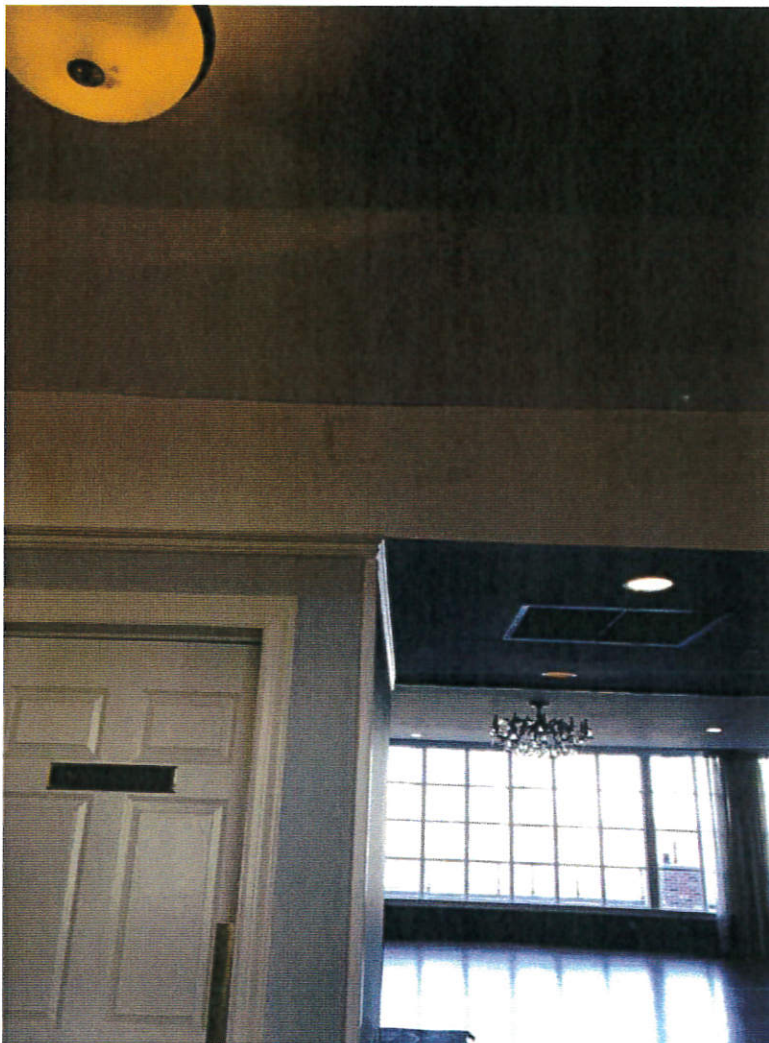
126 126-Pre-Mitigation - Foyer (Zone 2) Date Taken: 12/26/2022 9
