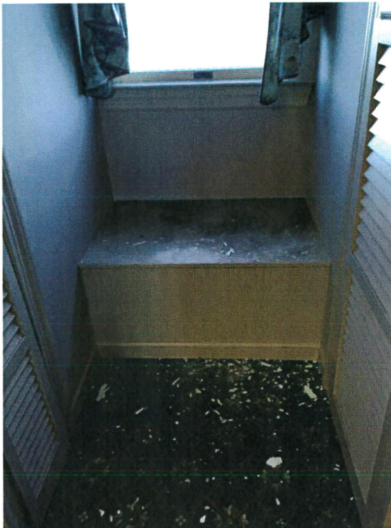
141 141-Pre-Mitigation - Locker room Date Taken: 12/26/2022 (Zone 1) 11
