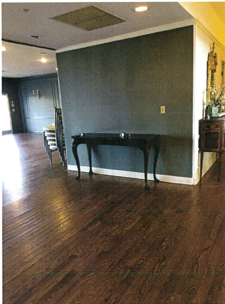
119 119-Pre-Mitigation - Foyer (Zone 2) Date Taken: 12/26/2022 2
