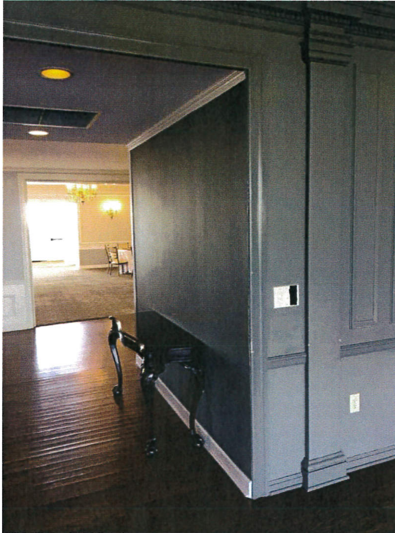
100 100-Pre-Mitigation - Ball room Date Taken: 12/26/2022 (Zone 2)
