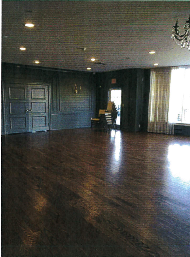
96 96-Pre-Mitigation - Ball room Date Taken: 12/26/2022 (Zone 2) 6
