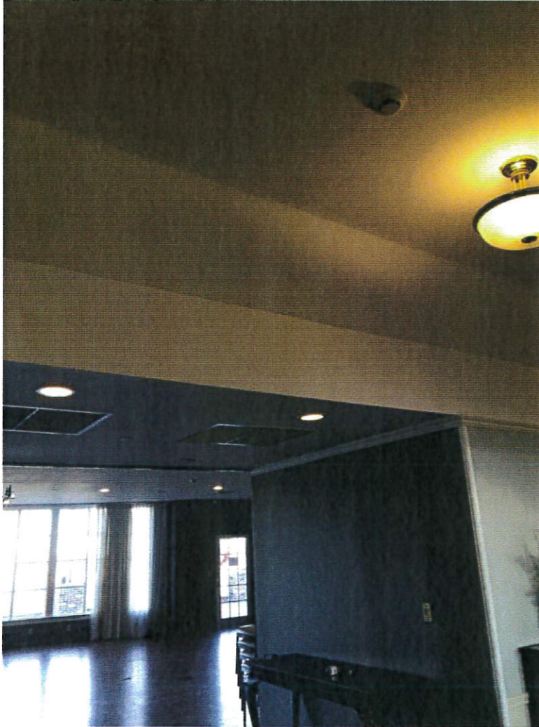
114 114-Pre-Mitigation - Foyer (Zone 2) Date Taken: 12/26/2022 10
