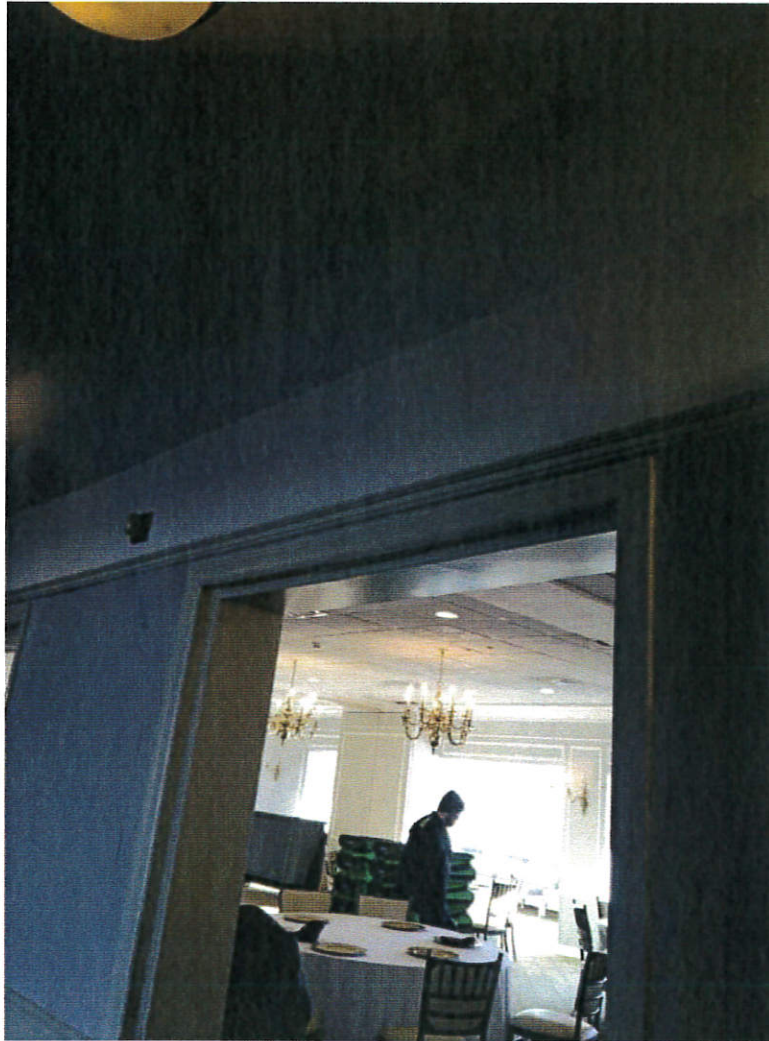
124 124-Pre-Mitigation - Foyer (Zone 2) Date Taken: 12/26/2022 7
