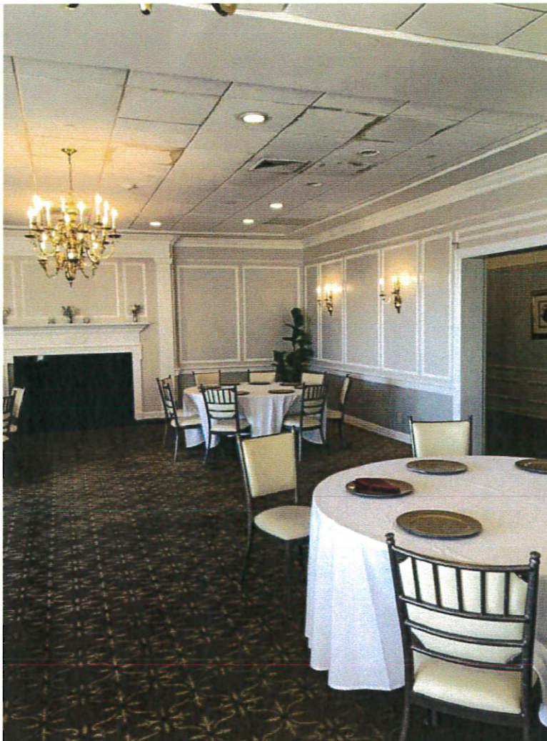
113 113-Pre-Mitigation - Dining Room Date Taken: 12/26/2022 (Zone 1)
