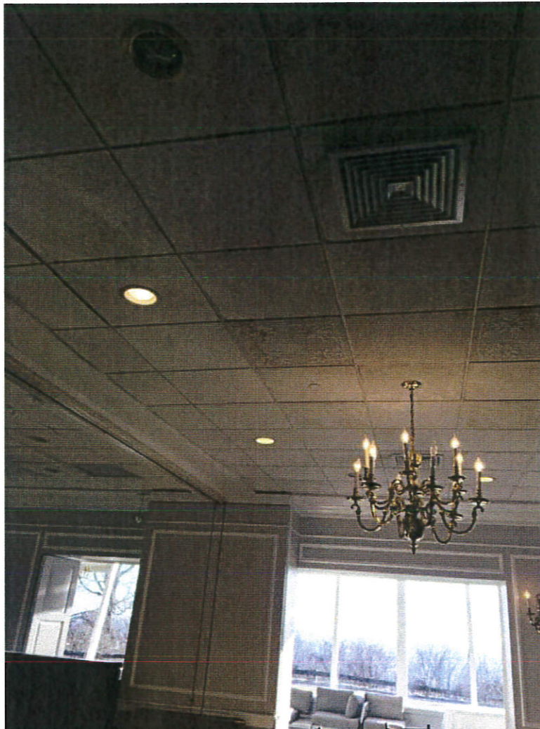
103 103-Pre-Mitigation - Dining Room Date Taken: 12/26/2022 (Zone 1) 12
