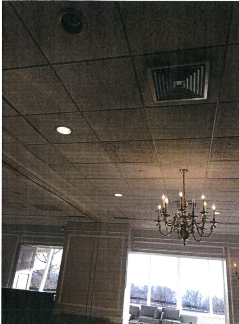
104 104-Pre-Mitigation - Dining Room Date Taken: 12/26/2022 (Zone 1) 13
