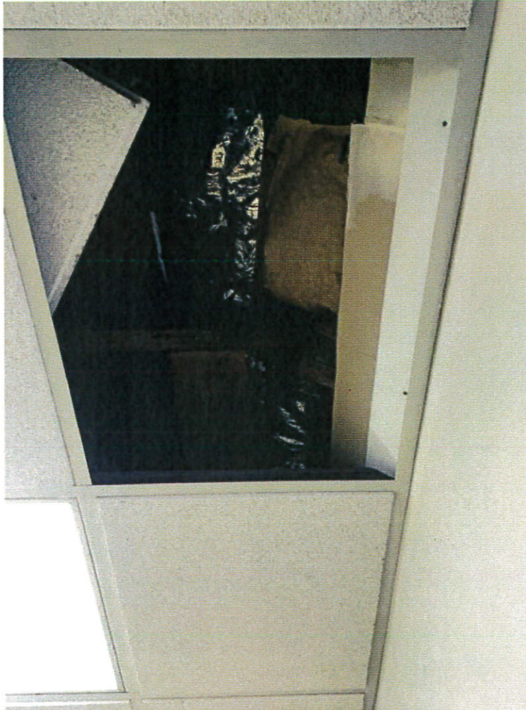
143 143-Pre-Mitigation - Locker room Date Taken: 12/26/2022 (Zone 1) 13
